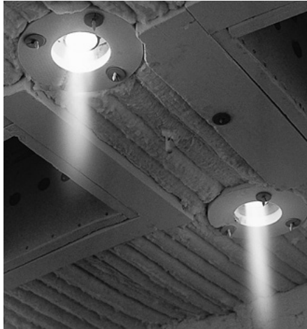
Overhead heating with burner BIC
